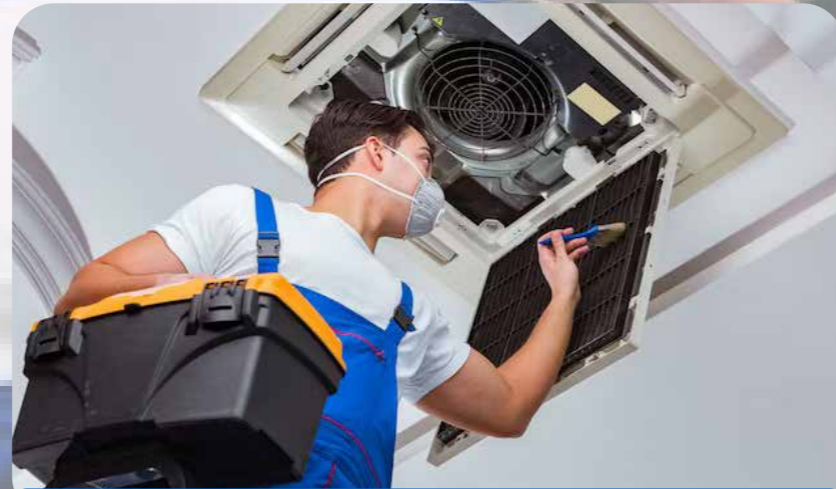
Air Conditioning Services
